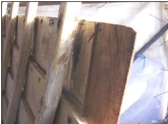
The first of many. This scarf had to run on the inside of the existing plank.
