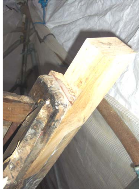
Replacement of much of the bow. This was glued and fastened with two stainless steel 10mm studs.
