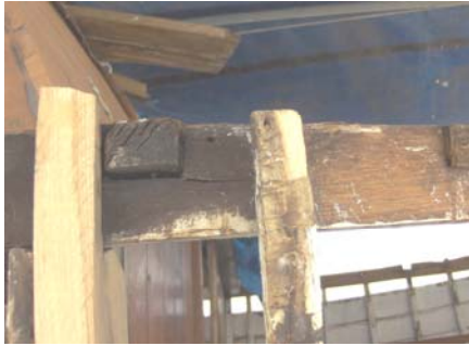
Rotten carling at the position of the mast head shroud. Note the frame, (left in the picture), under the mast had rot which was cut away and replaced with new oak.
