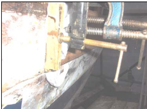
The scarfs were glued with West and then clamped, but not so tight as to squeeze the glue dry. Plastic bags were used to prevent gluing to the lower plank and the supporting block.
