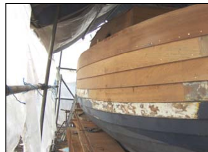
Continuing up the sides. The planks needed to be 24' long so I had to have a scarf mid-way, but staggered along the length.
